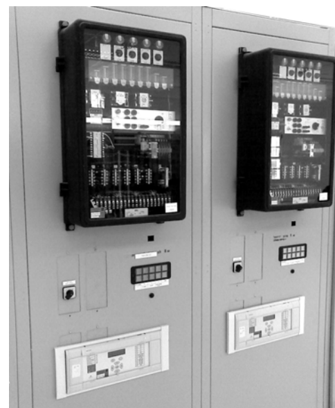
Fig. 1. Fragment of the protection panel at a distance of crucial lines 161 kV containing electromechanical relays of LZ31 type (above) included for working in parallel with an MPD type MiCOM P437 (below)
